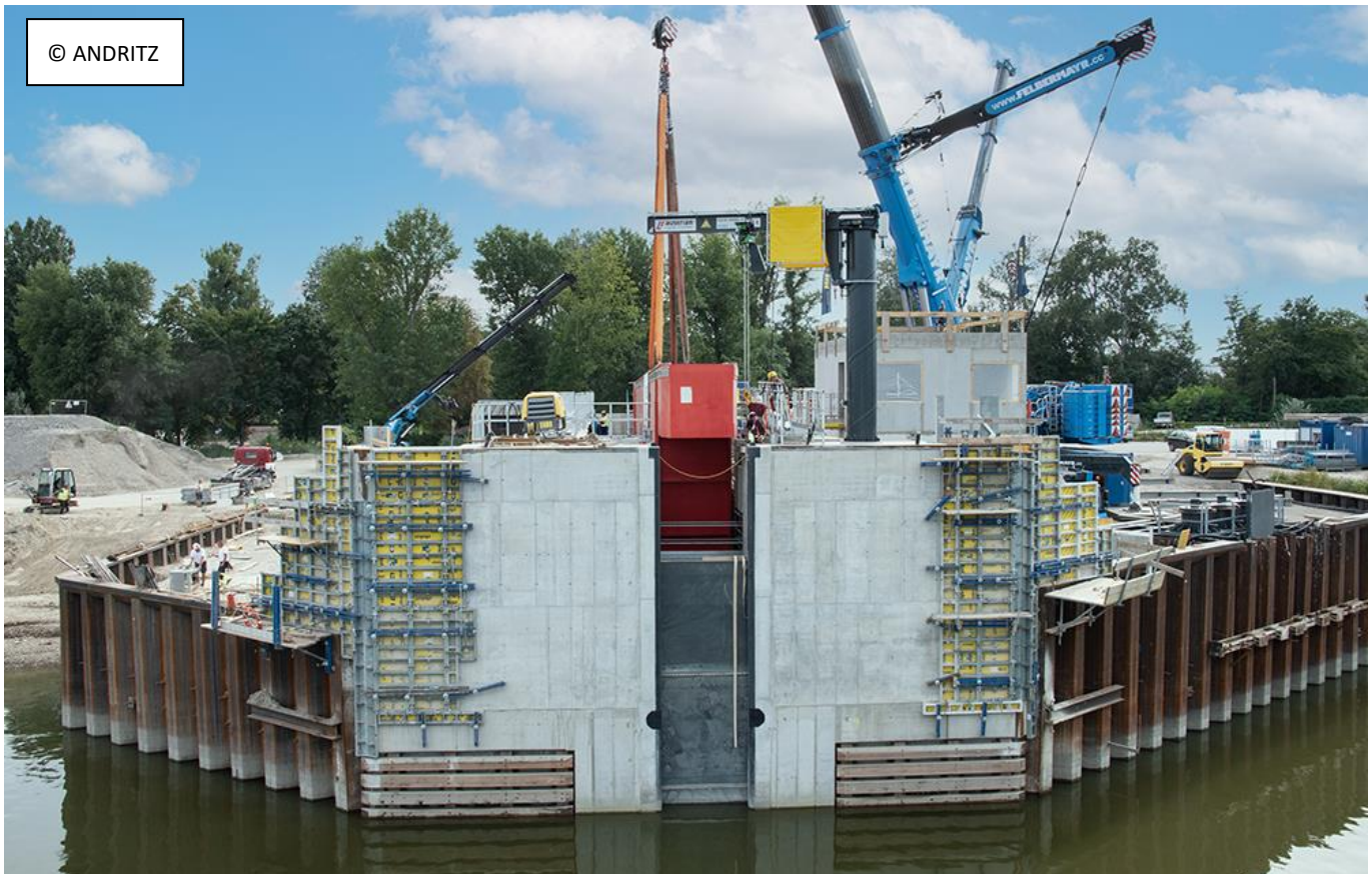
Figure 52: Sliding flood gate of the port of Albern.
