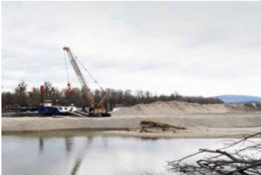
Figure 49: Creation of a new island improving the river dynamics in such a way that maintenance dredging in the navigation channel can be reduced or is no longer necessary. Source: viadonau.
